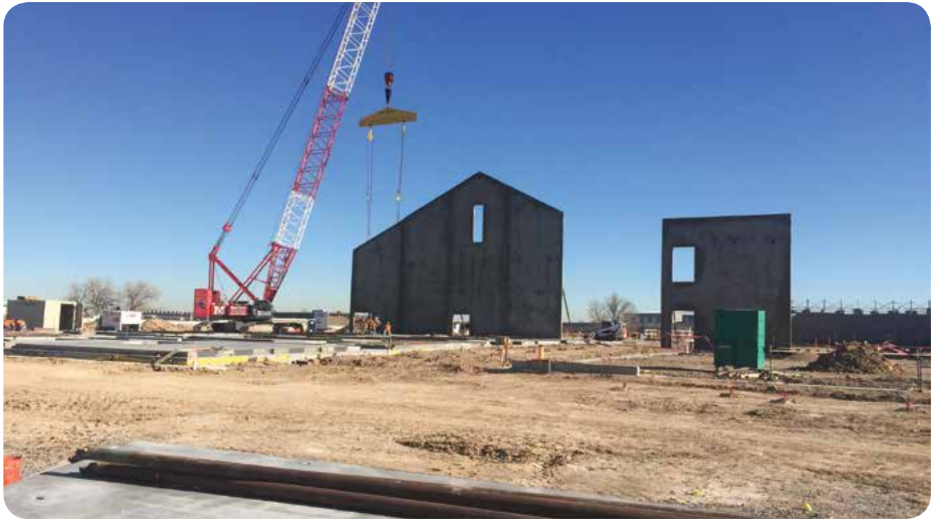
Crews raise the first of many concrete walls that are now in place at E. 112th Avenue and Potomac Street.
